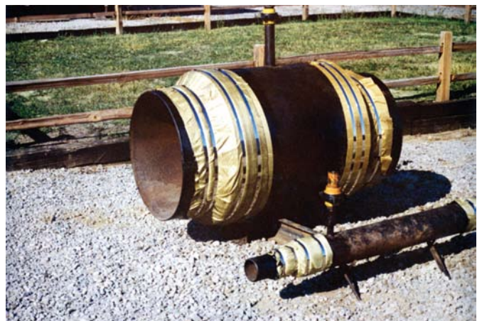
Two additional wraps of Seal-Wrap secured with two bands completes installation on small and large diameter pipes.
